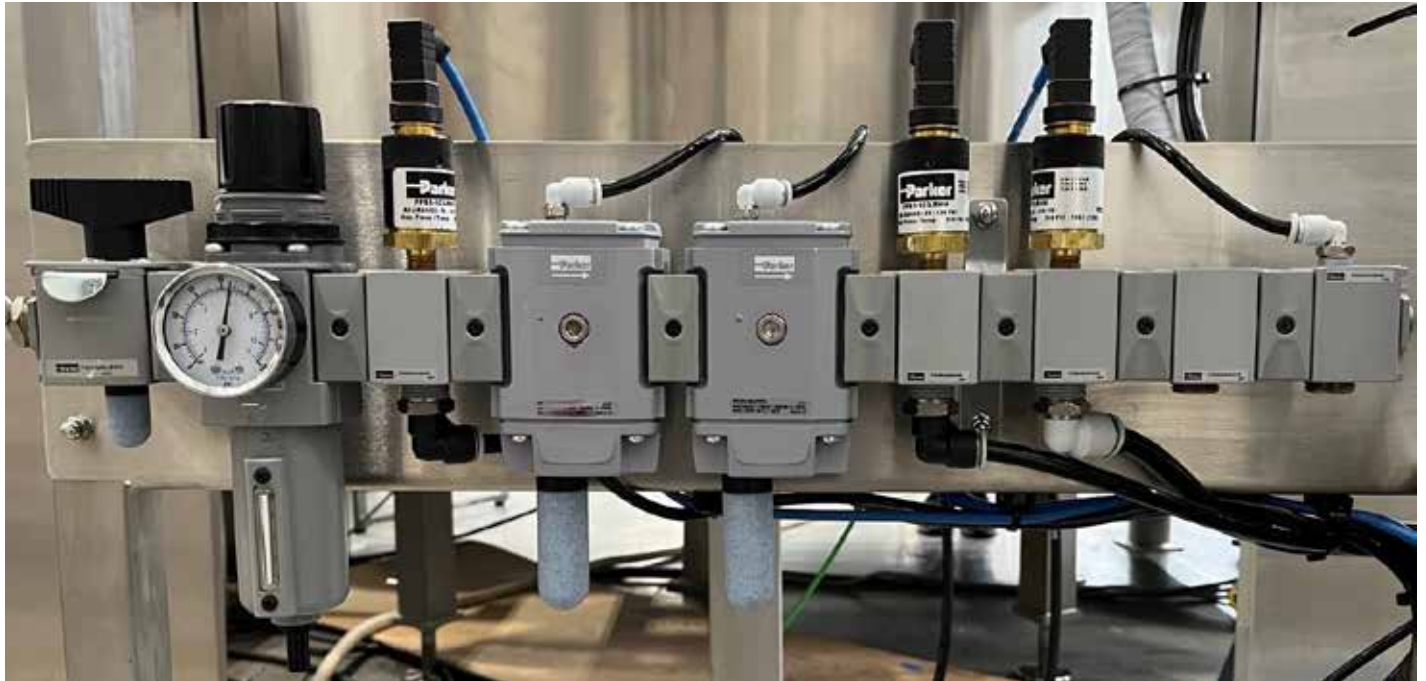
Figure 4-39: Air Prep Manifold Assembly
